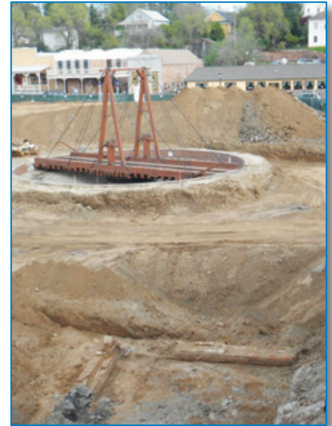
2011 excavation with Perkin's Warehouse foundation in foreground and historic turntable in background
